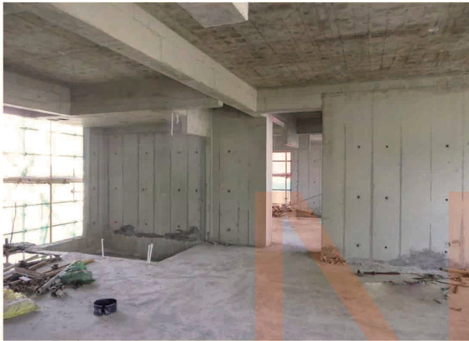
Interior wall formwork demoulding effect
